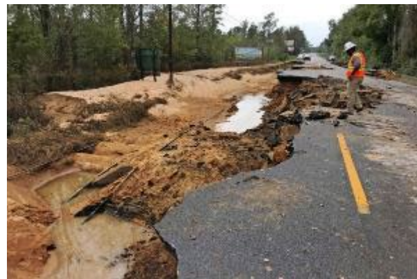
Figure 4-3. Flood damage to US 301 in South Carolina following Hurricane Florence in September 2018 (SCDOT, 2018).
