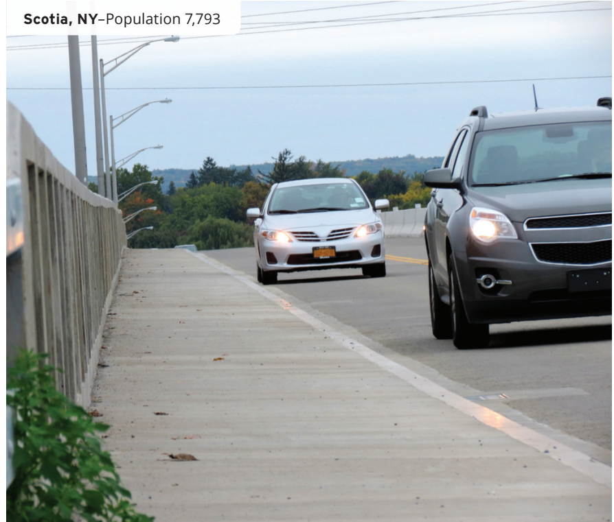
This sidewalk was installed over the existing bridge deck during a rehabilitation project.
